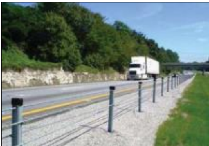
Figure 8: Wire Rope Safety Barrier
