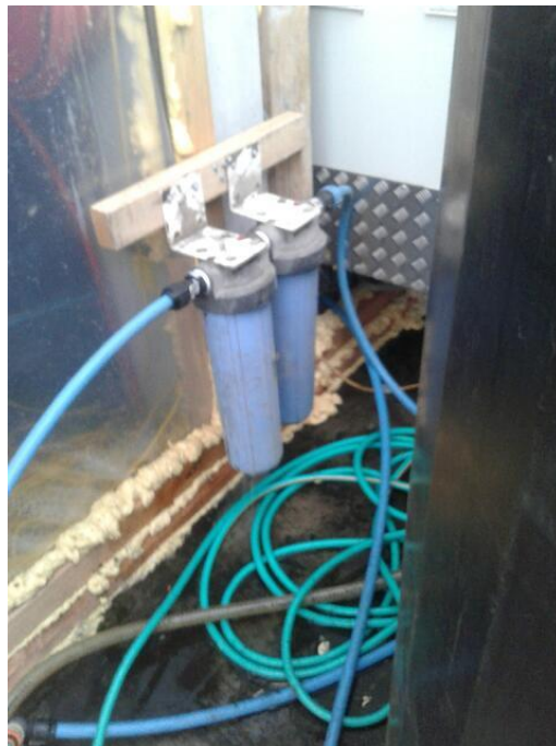
Figure 4: Double filtration water unit 20 to 1 micron capacity
