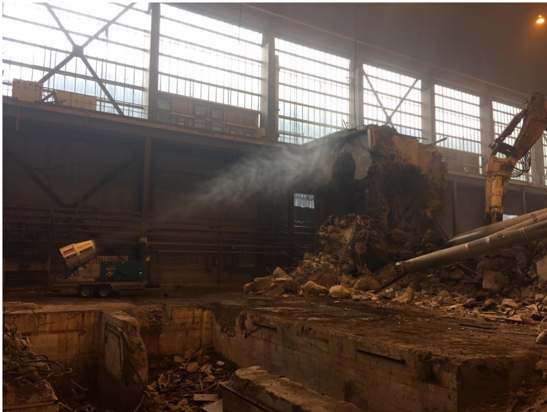
Figure 2: Water 11tomizer units.
