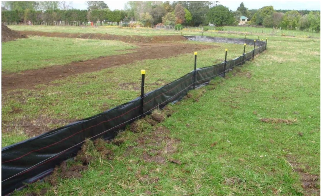
Figure 1: Example intended silt mesh protection to be installed to protect Maganone Steam
