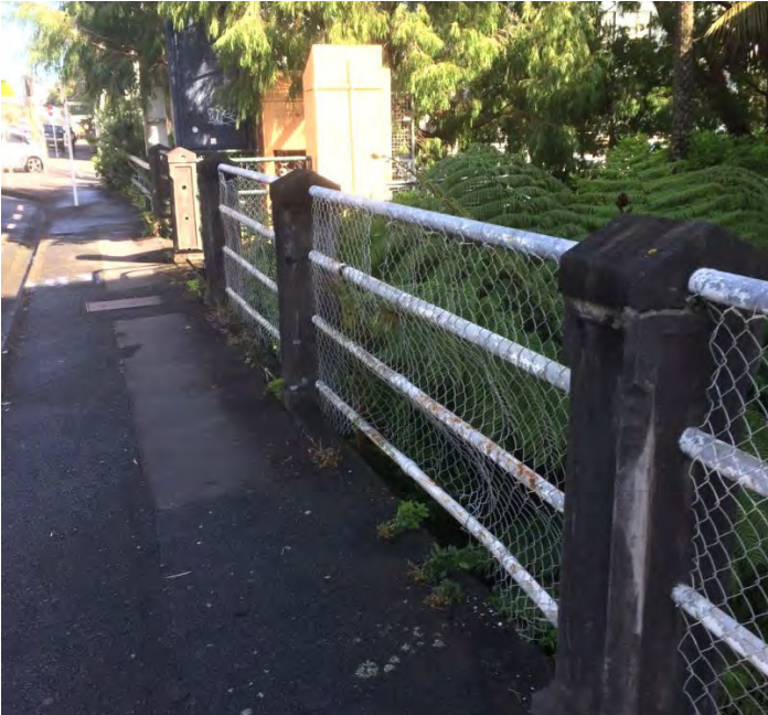
Plate 1 – Powderham Street Edge (Huatoki Stream overbridge and access to the Downtown Plaza)
