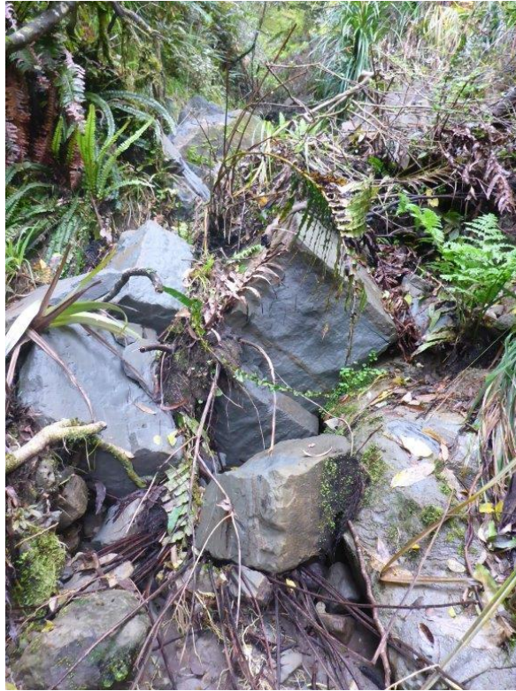
Figure 5: A recent slip of papa mudstone in ephemeral section upstream of site Ea15, Mangapepeke Stream (October 2017).
