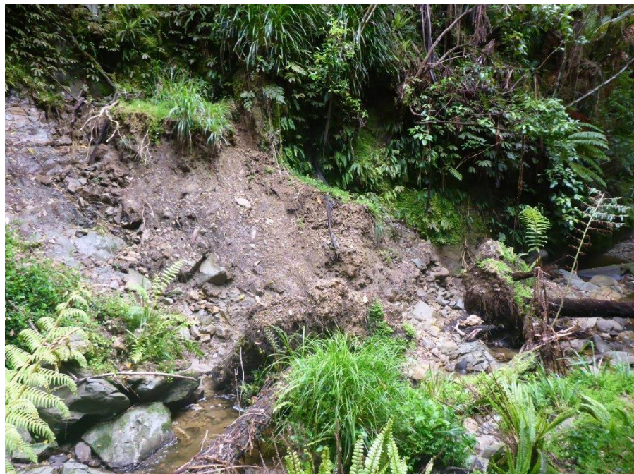
Figure 4: A small slip in the Mangapepeke Stream near site E5 (October 2017).
